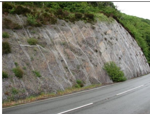
Fig.5. Gabion wire mesh used in keeping the possible fall of rocks and stones.
