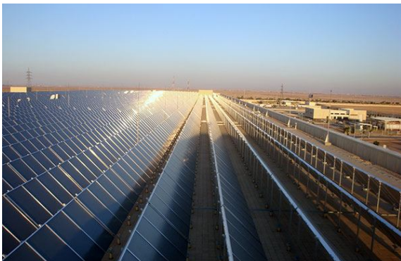
Figure 3: Solar panels at Princess Noura University
